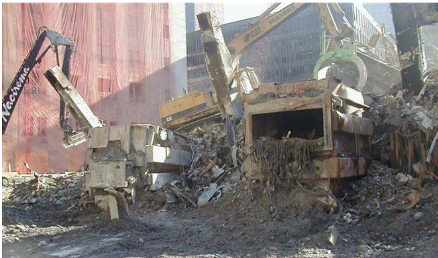
Figure A-8. Photograph taken in mid-October, 2001, showing Con Edison transformers #6 and #1 uncovered from debris pile of WTC 7.
