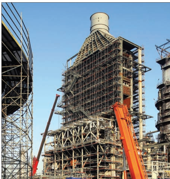
A new 125-megawatt cogeneration facility at ExxonMobil's Antwerp, Belgium, refinery is planned to start up in 2008, increasing energy efficiency of the plant.
