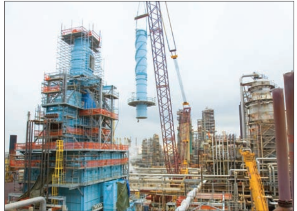
A new furnace stack is installed at ExxonMobil's refinery in Baytown, Texas, part of a project to increase capacity at a fraction of grassroots cost.
