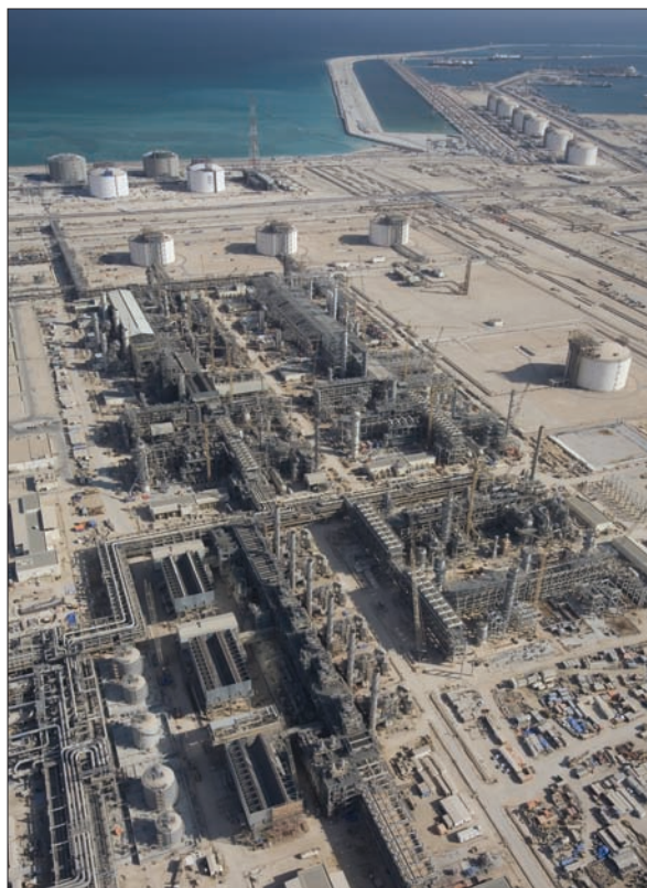
Construction on Qatargas II Trains 4 and 5 is advancing. These trains will export LNG to world markets utilizing the Port of Ras Laffan, shown in the distance.
