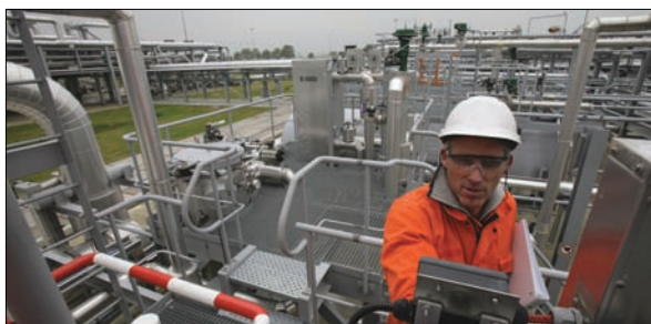
The giant onshore Groningen gas field is capable of producing up to 12 billion cubic feet per day to supply Europe's growing gas demand.
