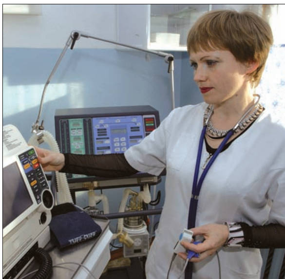
The DeKastri Hospital is one of the hospitals that was upgraded to manage medical and surgical emergencies within the community.
