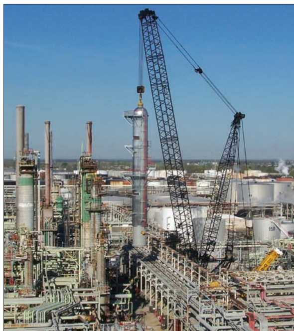
New facilities to reduce diesel sulfur were installed at our refinery in Baton Rouge, Louisiana, in 2007.
